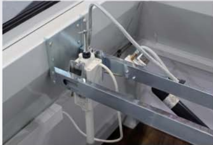
Electric drive for daily ventilation
