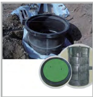
Infiltration rainwater well
