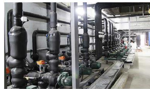
第比利斯-格鲁吉亚购物中心增压循环系统 PROJECT COMPLETE WITH BOOSTER SETS AND CIRCULATION SYSTEMS AT THE EAST POINT SHOPPING CENTER (TBILISI – GEORGIA)
